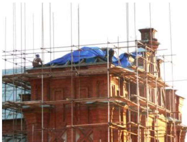
The scaffold is in place, and the old metal covers over the place for the steeples have been removed.
