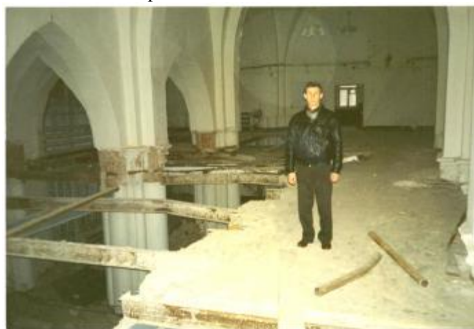
Trustee Andre Popok supervising the removal of the middle added floor in the church.
