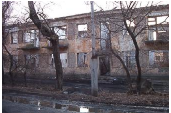
The ruins of an old apartment building that was at first considered as possibly suitable to remake as a church. The specialists say that the bricks have been too ruined by water and freezing to use again as a building.
