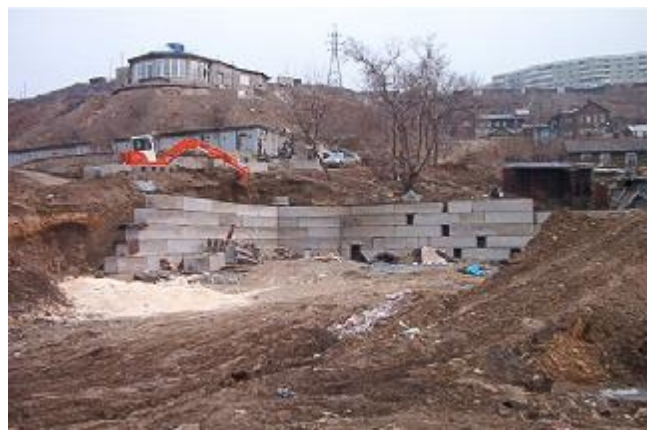
Construction continues on the Our Lady of Fatima rectory in Vladivostok, in spite of the cold weather.
