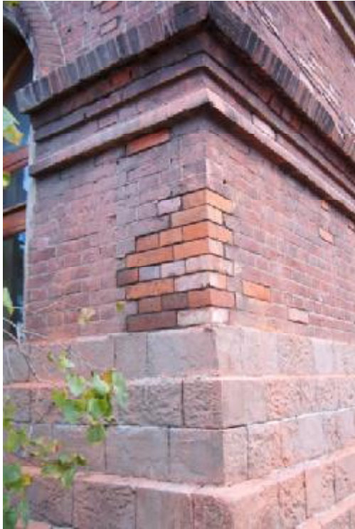
After work on the bad corner. The whole wall has still to be worked over for uniform color.
