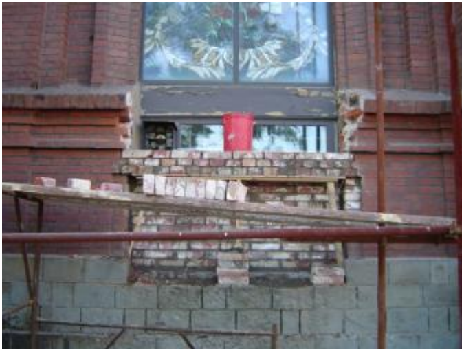
The extra windows broken into the outside walls on the South side have to be reclosed, so that the building, an architectural monument, will look as it did when it was built from 1908-1922.
