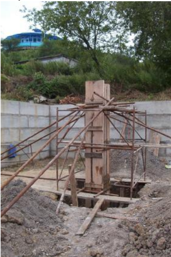
The first pillar of the two-storey building and basement is rising toward the sky.
