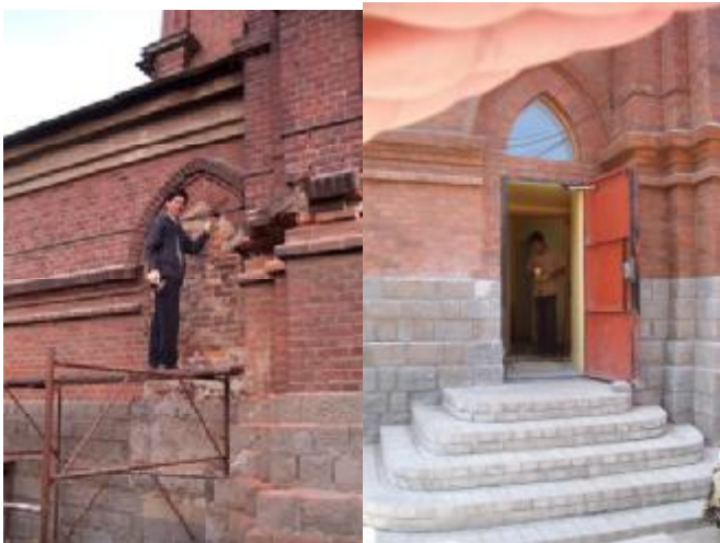
Remember this old bricked-up door? Here it is now—the main door to the sacristy.
