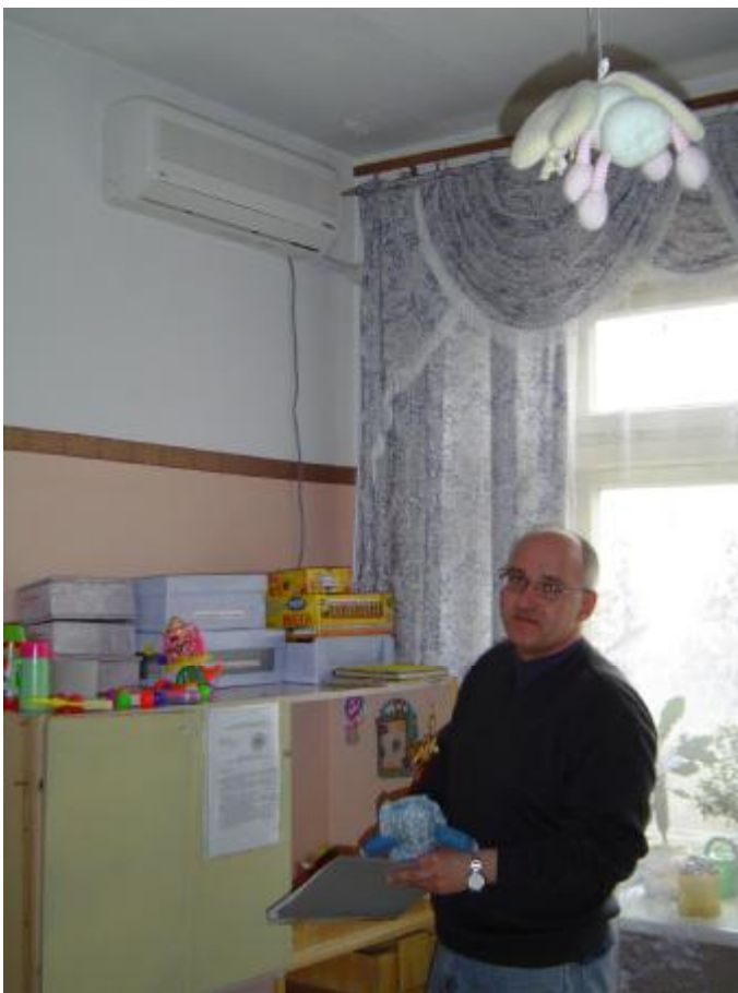
Denis Bondaryev of St Vincent de Paul in Vladivostok who oversaw the air conditioners' installation. One of the inside units is visible overhead.
