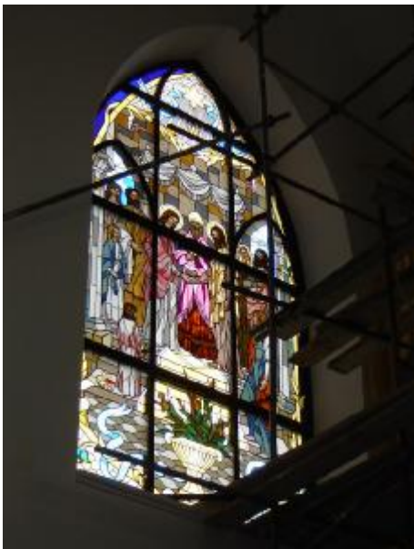
Two windows in the process of installation: "The Marriage of Mary and Joseph" Donated by Mr and Mrs Robert Ozburn
