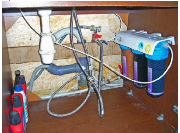
Repairs were needed in the kitchen, too.
