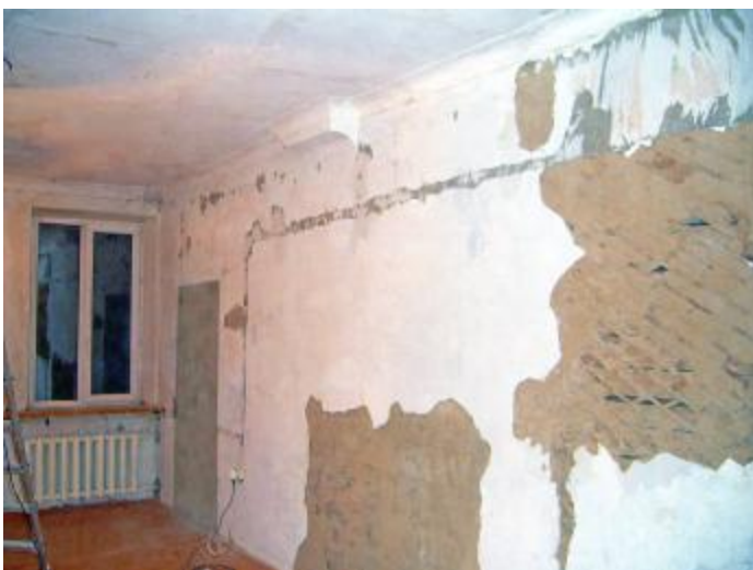
Wall to be repaired in Nakhodka's chapel.
