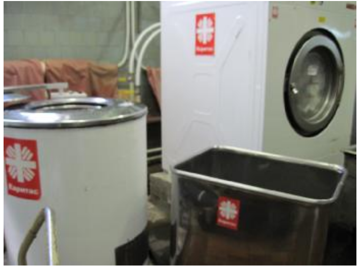
Equipment installed in Hospital #3
