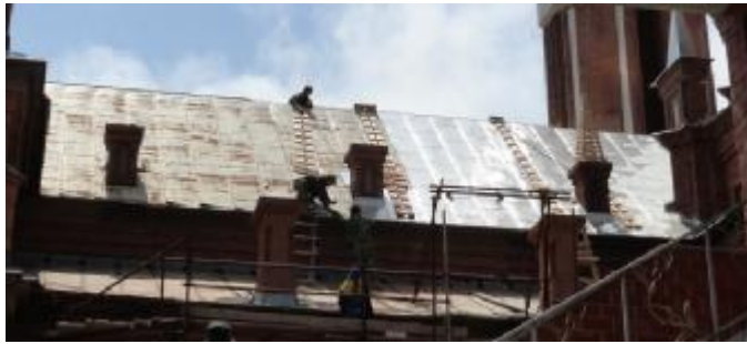
Old roof to the left; new roof to the right. Don't fall, please!
