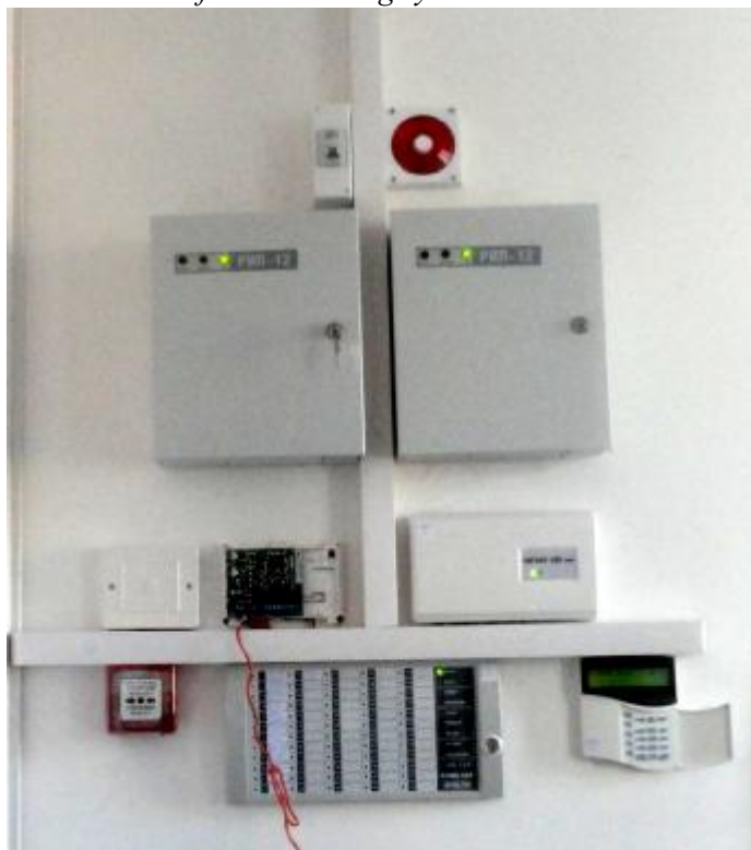
The automatic fire monitoring system
